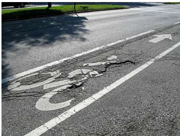
Figure 10.5 – Poorly Maintained Bicycle Lane
