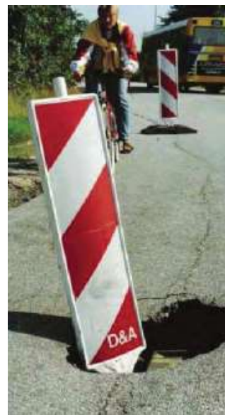
Figure 10.10 – Pothole Identified by Hazard Marker
